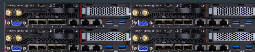
Side by side in rack
